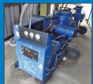
(2) 25 HP Quincy QSB-25 Air Compressors
