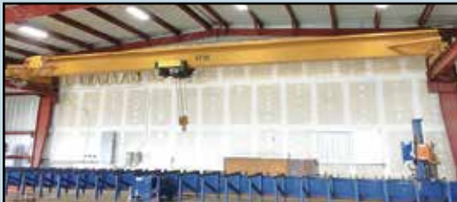
5-TON CRANE W/60' SPAN, 65' OF PAIRED RUNWAY
